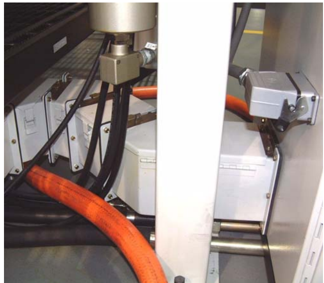
Machine Base Connections
